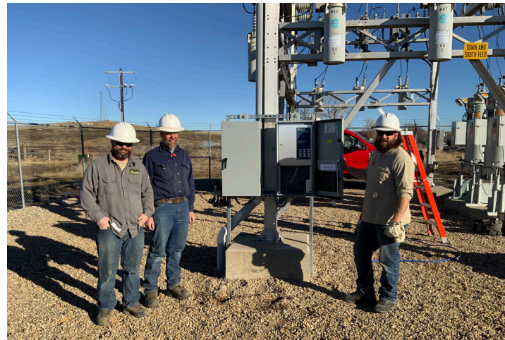
ABOVE: (L-R) Lineman Jake Grensten, Apprentice Lineman Jason Deffinbaugh and Transformer Repairman Mark Schwomeyer perform maintenance at the Winnett Substation.
