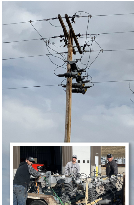
(L to R) Dan Rice, Lineman; Travis Sura, Apprentice; Bill Stanton, Lineman are ready to head out to the field to install three-phase Compact Modular Reclosers
